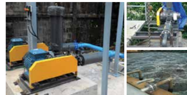
1. Water Treatment System
