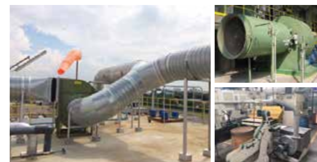
7. Supply and Exhaust Air System
