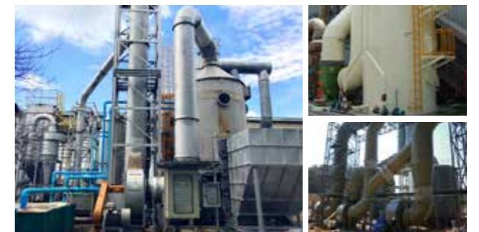
2. Wet Scrubber System
