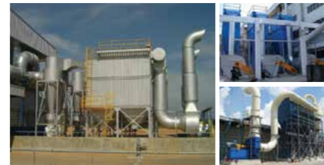
3. Dust Collector System
